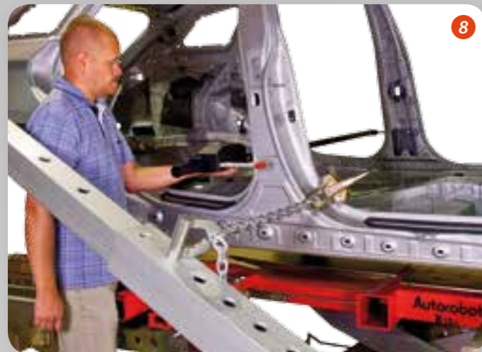
Autorobot B15 Super is perfect for various jobs in car body shop. Picture 8 shows the straightening of B-pillar under guidance of EzCalibre electronic measuring gauge.
